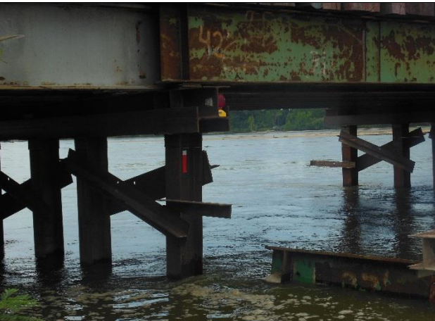
September 4, 2015 – Photo showing flashing light and reflective tape on upstream side of bent row #2.
