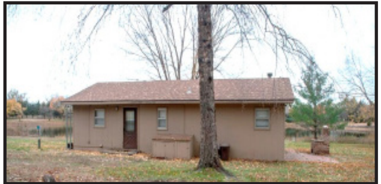
HOMES LIKE THIS ONE IN CEDAR CREEK HAVE THEIR FIRST FLOOR 4 OR 5 FEET BELOW THE BASE FLOOD ELEVATION. ELEVATING THIS HOME WOULD REDUCE FLOOD AND FLOOD INSURANCE, AND MAKE THE FAMILY SAFER.
