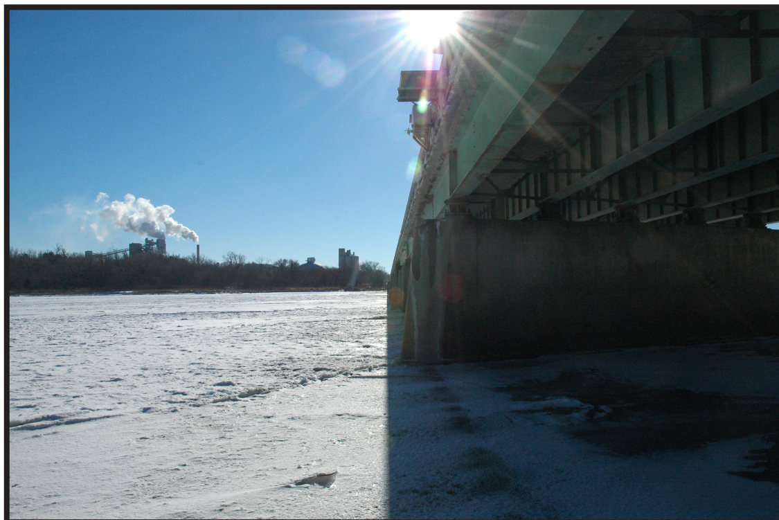
Louisville, NE in the distance as seen from under the Hwy 50 bridge photo by Josh Price
